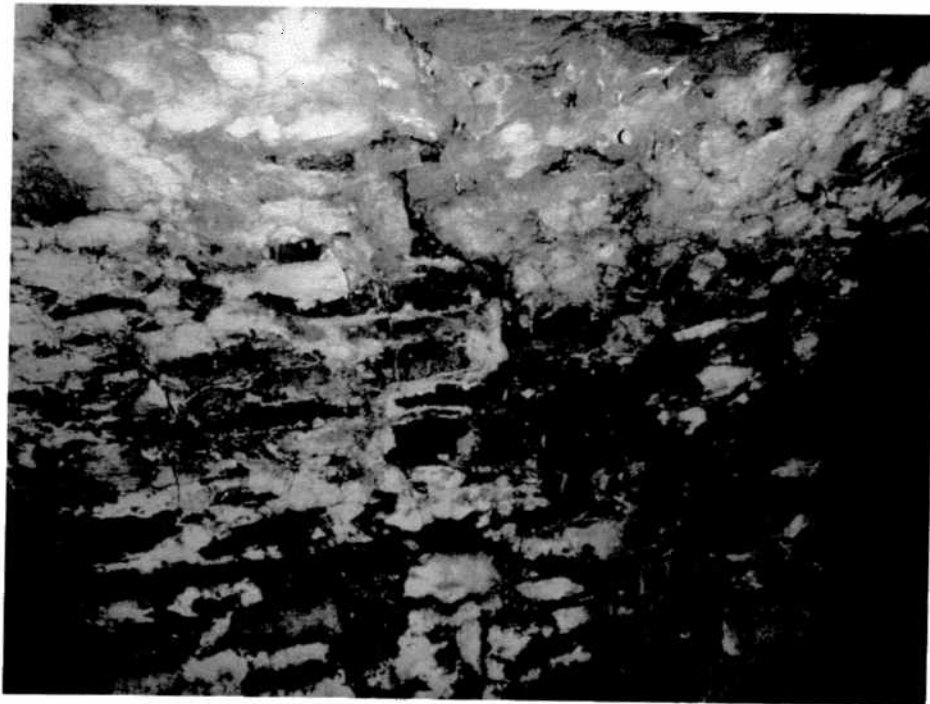
Photograph 4. Wide crack in West Wall ↑
