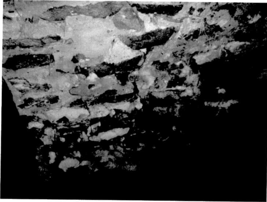
Photograph 7. Loss of Mortar from Stones!↑
