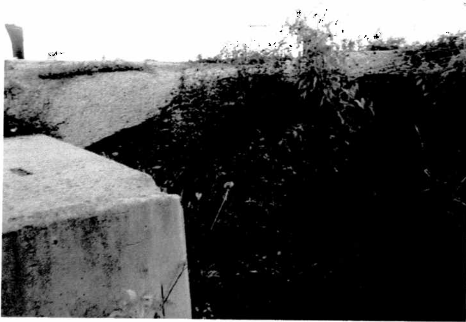
Photograph 5. Severe Erosion of Southeast Embankment ↑
