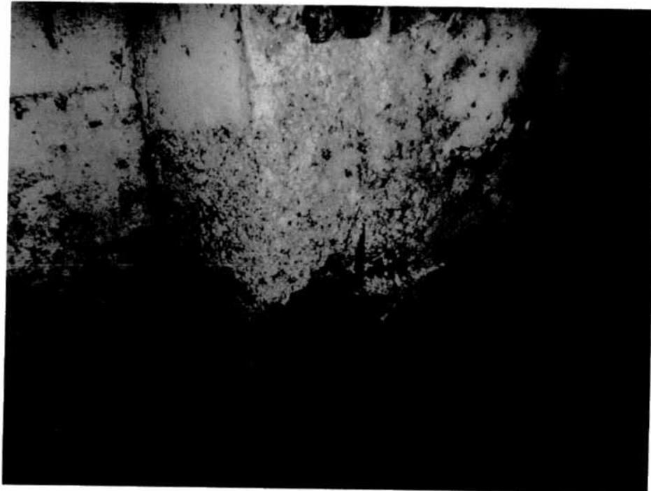
Photograph 2. Light Honeycombing of Barrel Wall ↑
