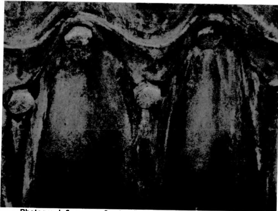
Photograph 6. Crack at Bolt Hole Location in Culvert Wall ↑
