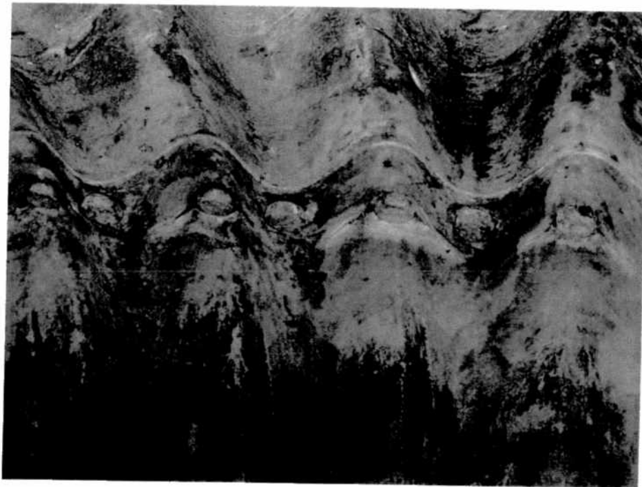
Photograph 4. Crack at Bolt Hole Location in Culvert Wall ↑
