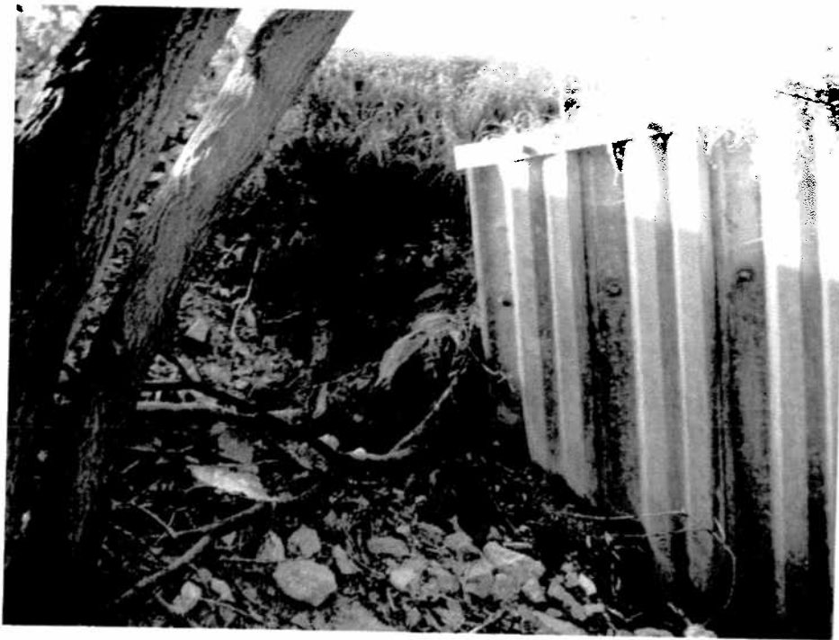
Photograph 4. Minor to Moderate Erosion of Embankment in Northeast Quadrant ↑
