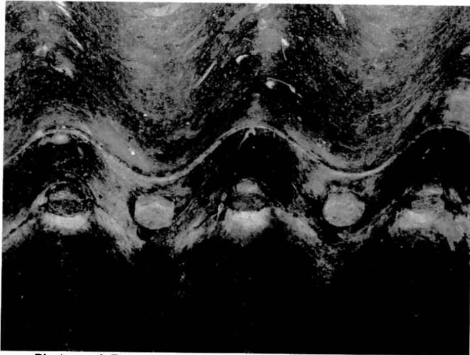
Photograph 7. Crack at Bolt Hole Location in Culvert Wall ↑
