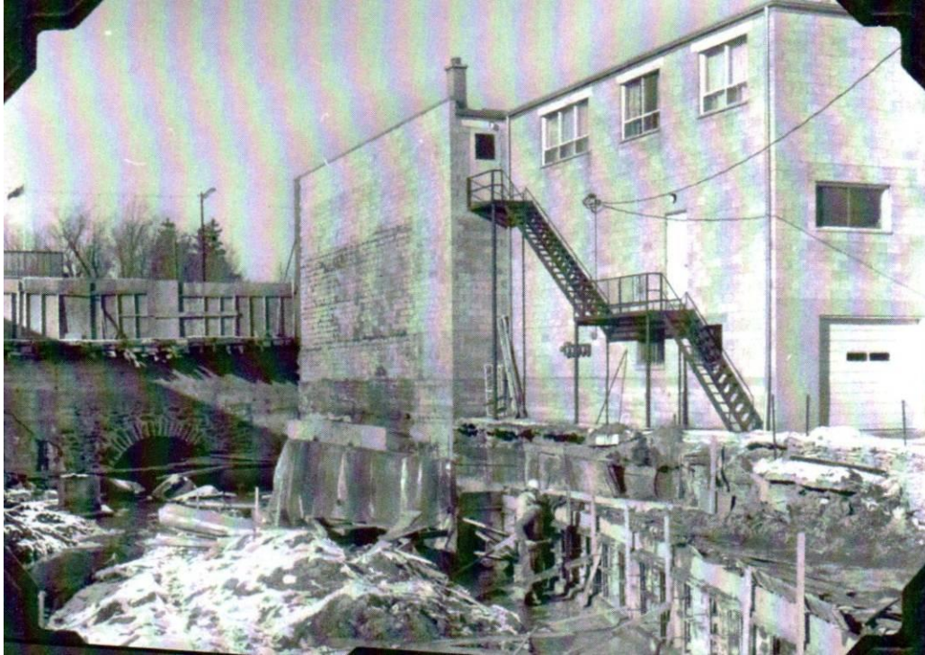
Image 3: Looking north at construction activities during installation of culvert immediately south of Brock Street, November 1972. The building to the right still exists today (see Image 6 ) (Courtesy of Uxbridge Public Library)
